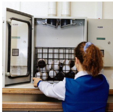
A receive cabinet in the cash office
