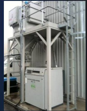
Typical exhauster plant
